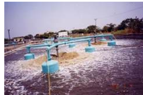
Slow Speed Floating Aerator
