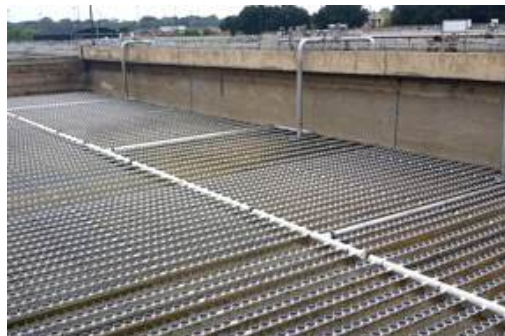
Diffused Aeration System
